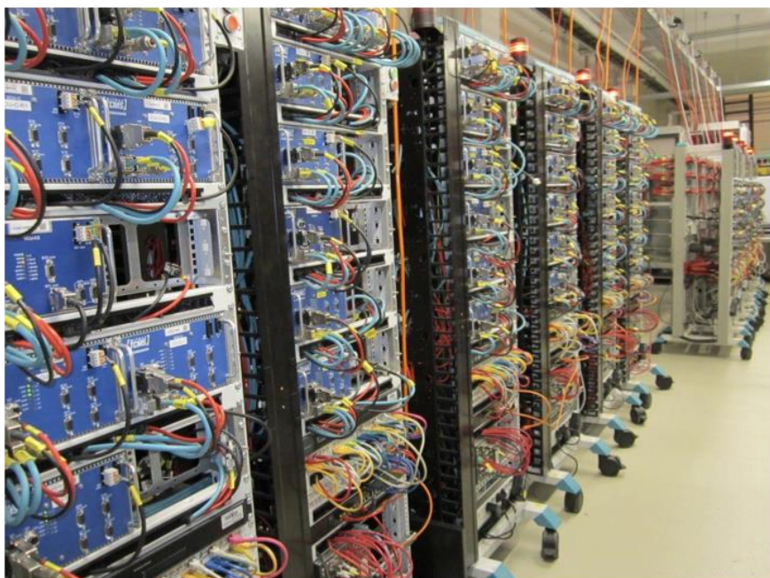
Figure 11. TCMS Test Racks.
